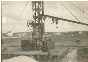
Mechanical equipment at the port of Argenton
